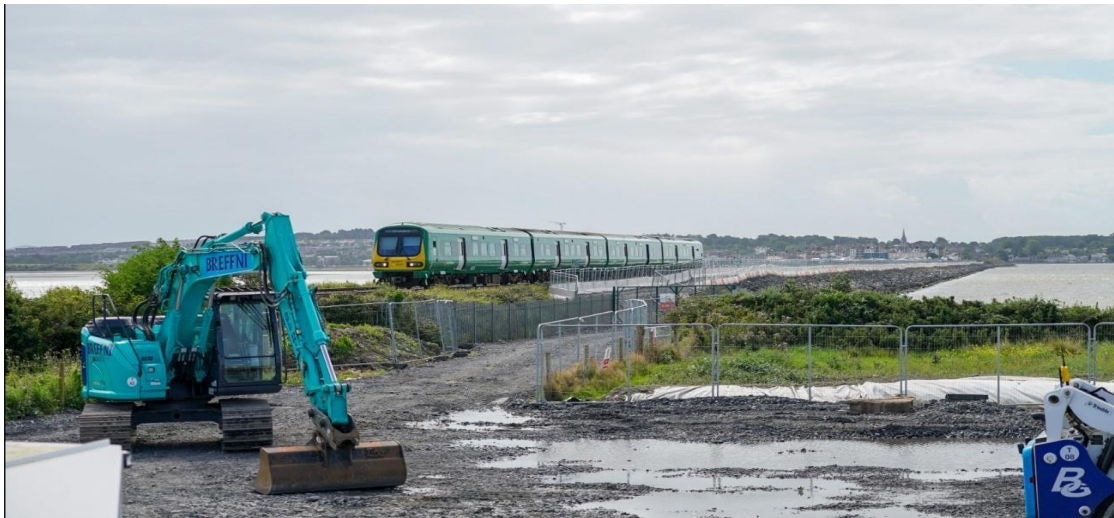
Fig 4. Building on the initial haul road, Fingal Co Council commenced a project to extend it across the Estuary and on to Donabate as a walkway/cycleway. Started in late 2023 by building a haul road, it will be completed in early 2026. (Irish Times Picture August 2023)
